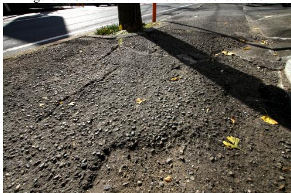
Figure 3. The old pavement on the sidewalk
