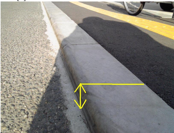
Figure 1. Sharp drop in the level of the road
